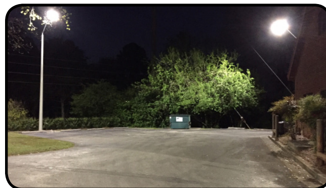
Pictures shown are of our parking lot lighting before and after the conversion.
